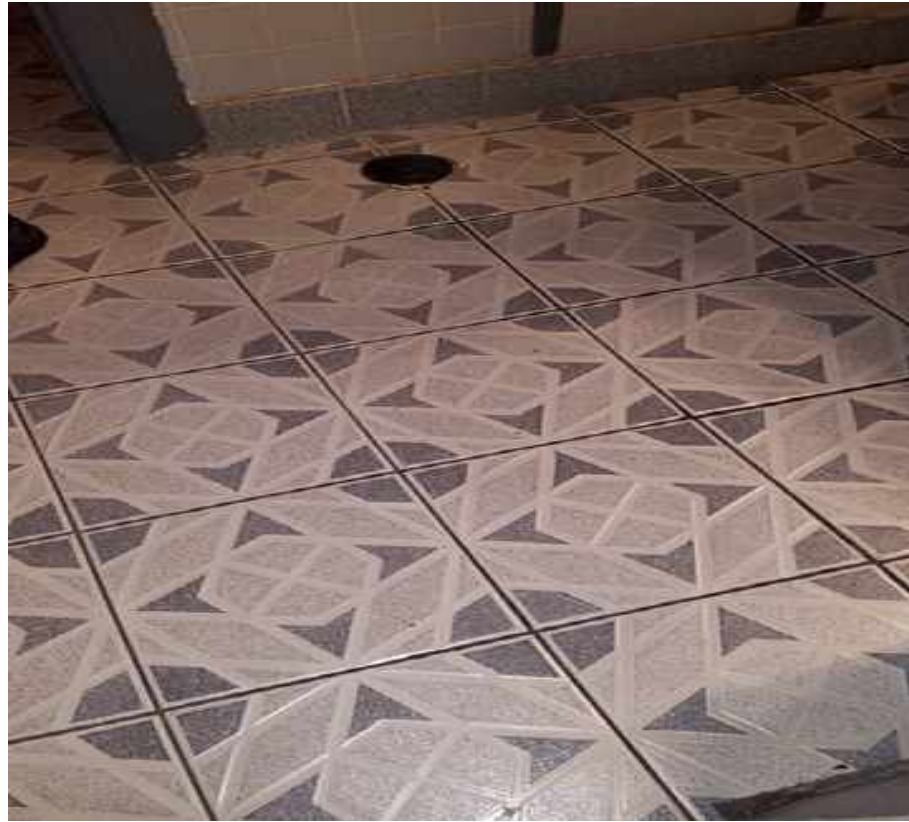
47. Gemmell's Restaurant. Lead-based ceramic floor tile in Men's restroom.
