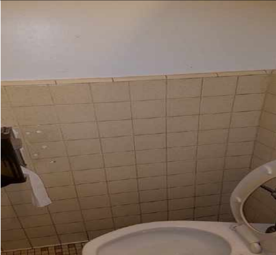
42. The Brig Restaurant. Lead-based beige ceramic wall tile in the employee restroom,
