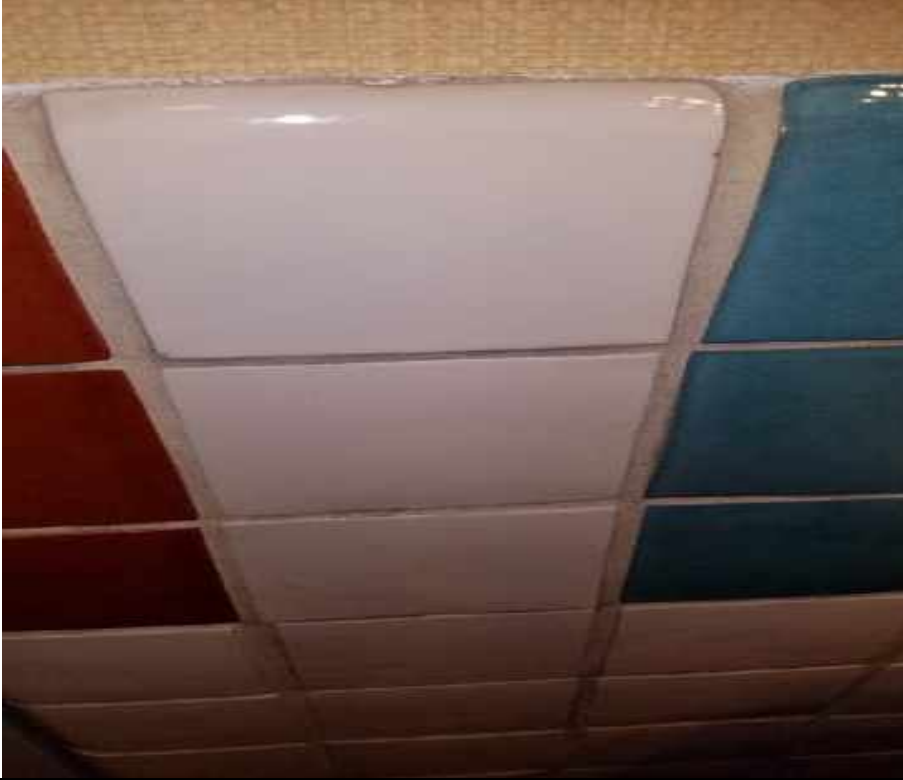
51. Harbor Grill Restaurant. Lead-based red, blue and white ceramic wall tile in the restrooms.
