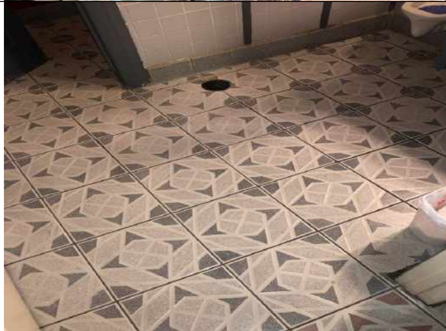
30. Gemmell's Restaurant. ACBM flooring mastic (under ceramic tile).
