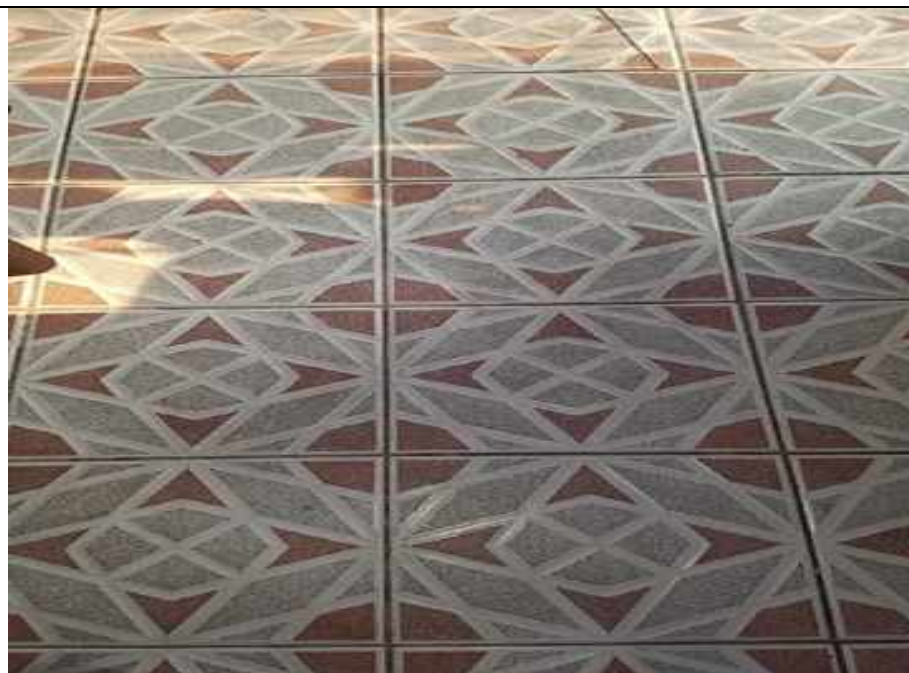
48. Gemmell's Restaurant. Lead-based ceramic floor tile in the patio dining area.
