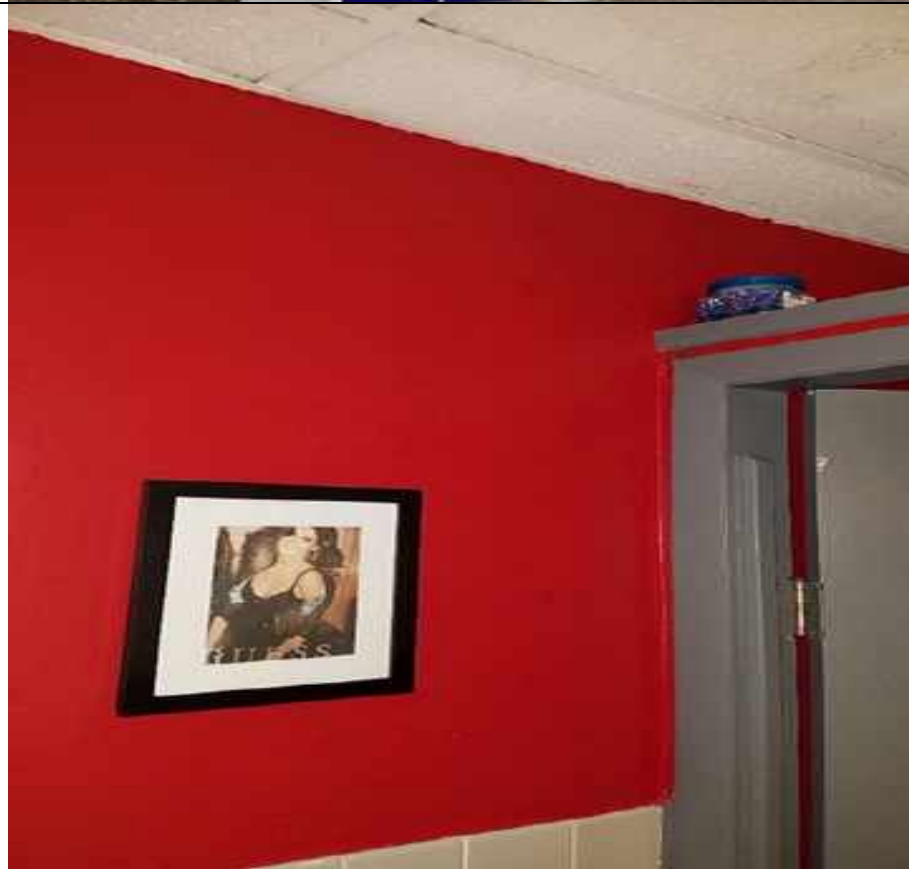
46. Gemmell's Restaurant. Red lead-based paint on drywall.
