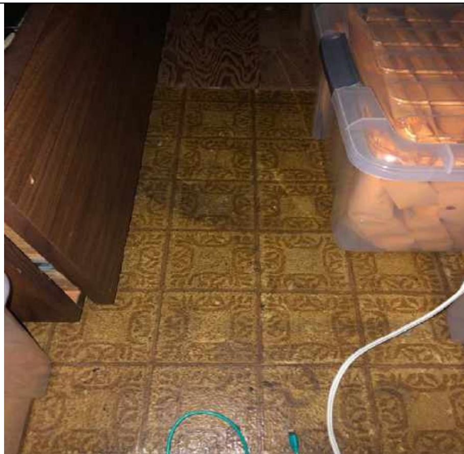
38. Wind & Sea Restaurant. ACBM vinyl sheet flooring.
