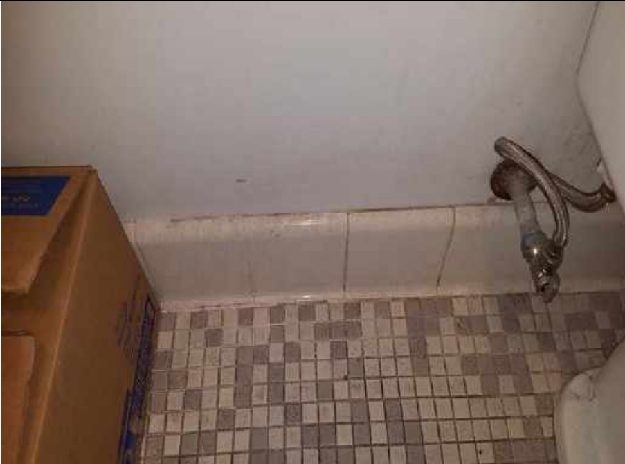
52. Killer Dana. Lead-based white ceramic wall base in the restroom.
