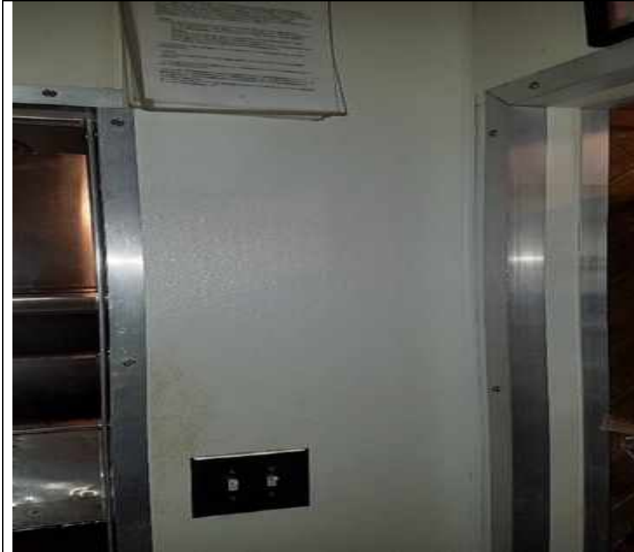
54. Turk's Restaurant. Lead-based painted wall covering in the kitchen.
