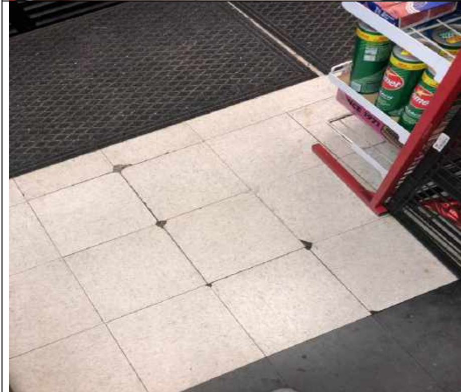
26. Village Market. ACBM white 12" vinyl floor tile.
