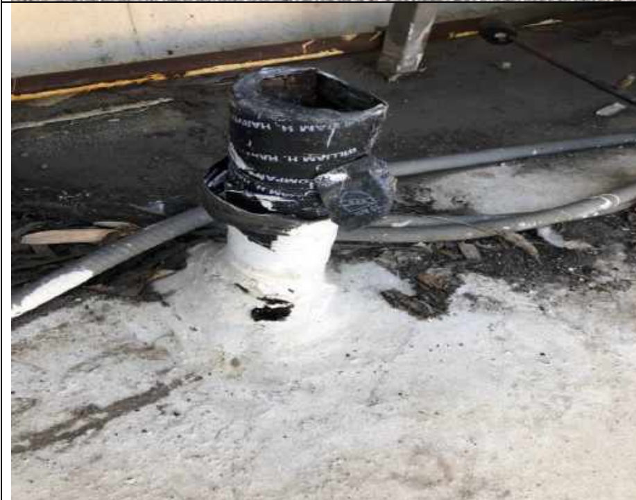
34. Harpoon Henry's Restaurant. ACMB roof mastic.
