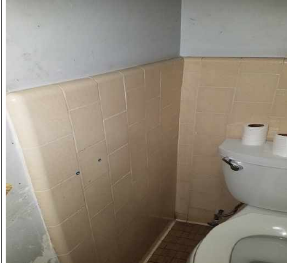
43. Dana Wharf Sportfishing. Lead-based beige ceramic wall tile in the Men's restroom.
